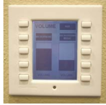
The Crestron touchpanel is interfaced with the Intelix MARC room combine system, allowing facility users to control audio source selection and volume.
